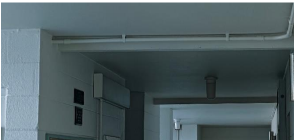
Fig 3.3 Hallway lights – 1 st floor
