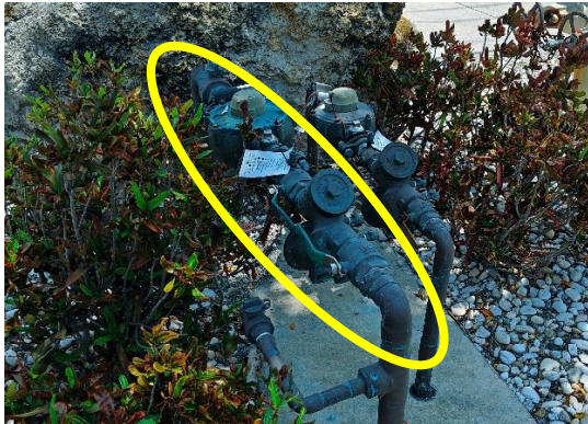
Fig 7.1 Main water valve to building
