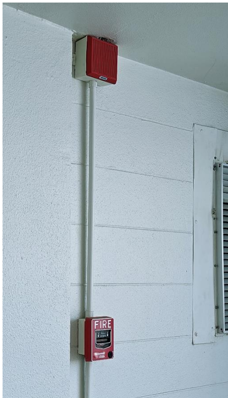
Fig 12.5 Fire alarm pull & horn
