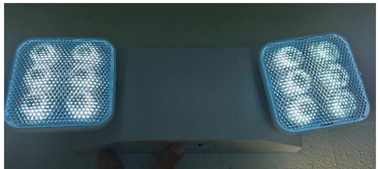
Fig 12.7 Emergency lights turned on
