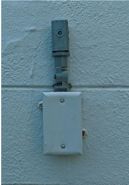
Fig 5.2 Sensor to turn on & off carport & main entrance lights
