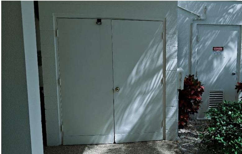
Fig 11.5 Elevator room door on right & key box on left
