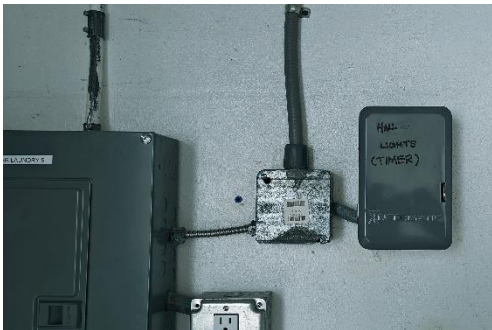
Fig 3.1 Hallway light timer box – 5 th floor laundry room
