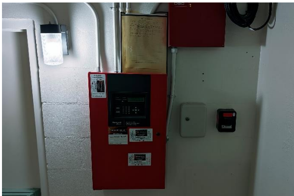
Fig 12.1 Fire panel cabinet
