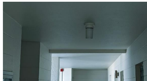
Fig 3.4 Hallway lights – floors 2 - 5
