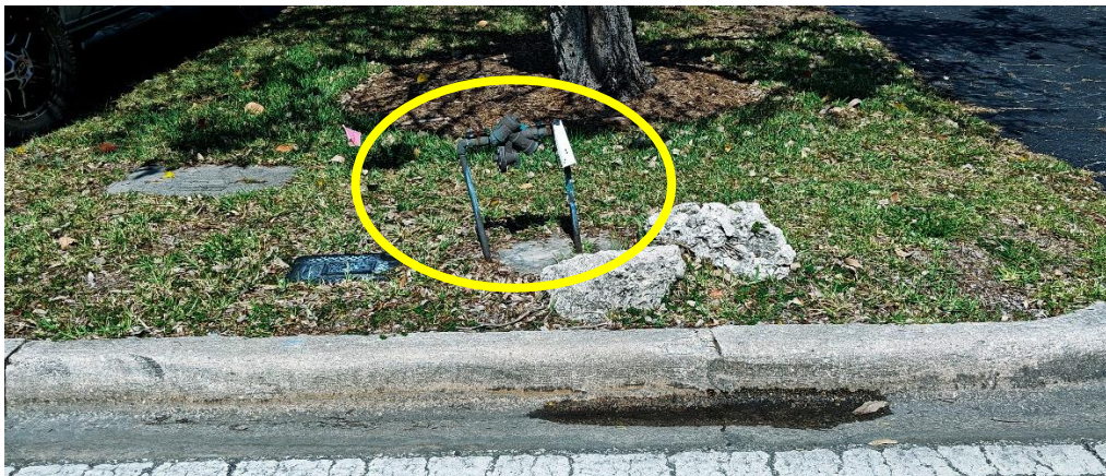
Fig 9.3 East side irrigation water shutoff valve
