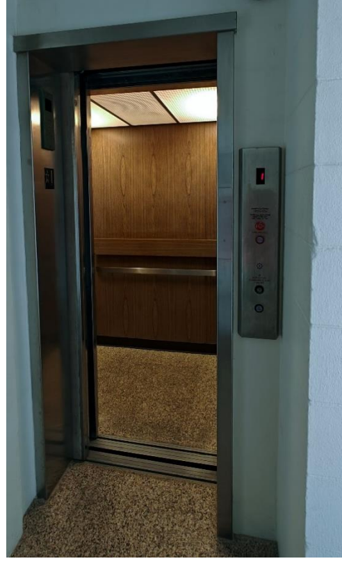
Fig 11.4 Inside elevator cab
