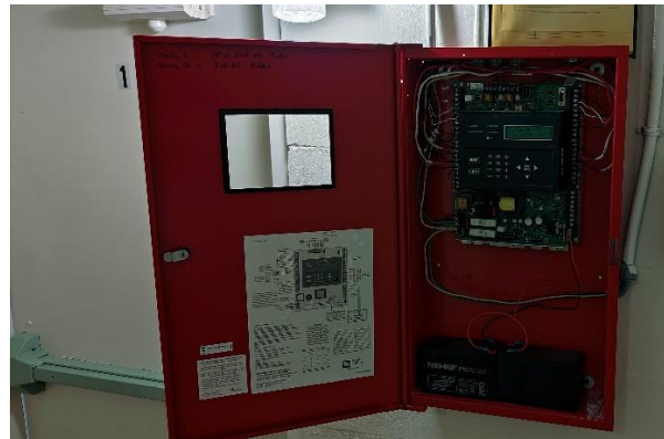
Fig 12.2 Fire alarm panel
