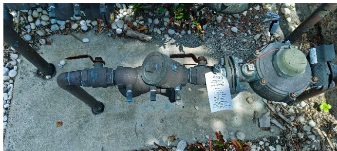
Fig 8.4 Beach water and west side irrigation water shut off valve – top view
