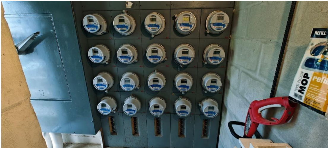
Fig 2.1 Unit electric meters in electric room
