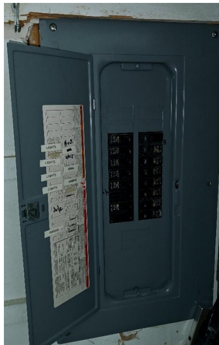
Fig 2.2 Electric panel in individual unit
