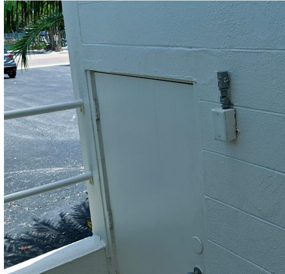
Fig 5.3 Sensor to turn on & off carport & main entrance lights by electric room door
