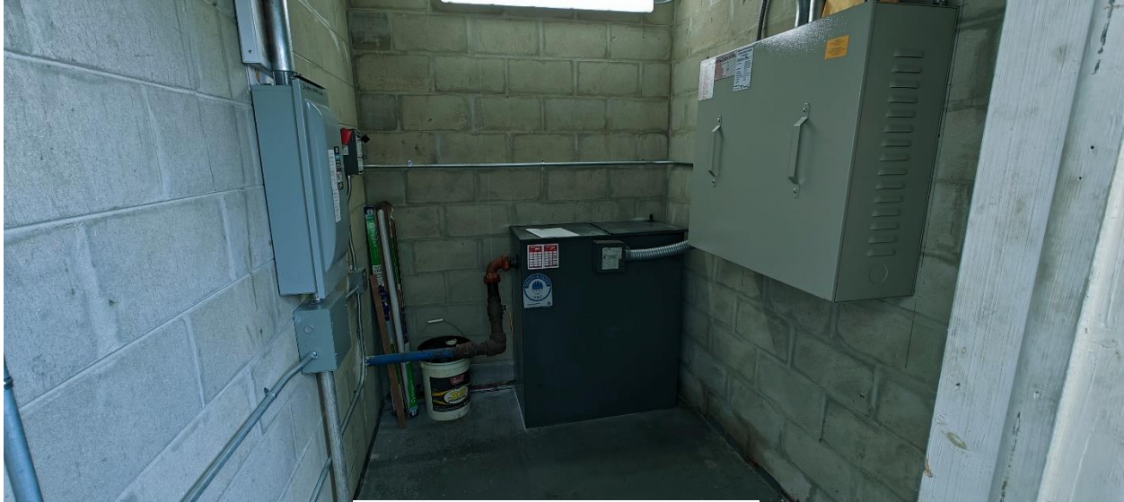
Fig 11.7 Inside elevator room
