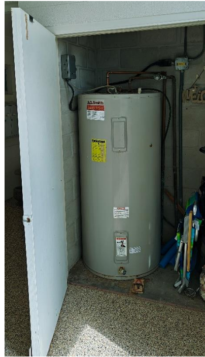
Fig 4.2 Laundry water heater
