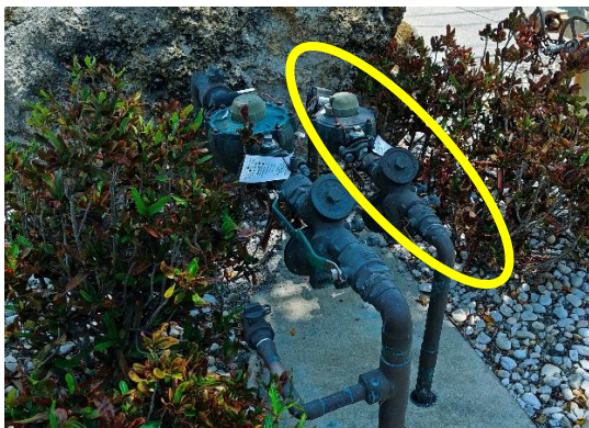
Fig 8.3 Beach water and west side irrigation water shut off valve
