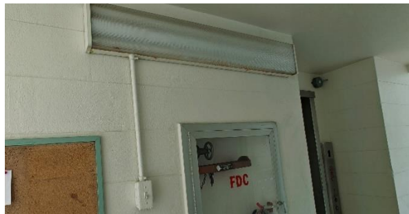
Fig 3.5 First floor fluorescent light
