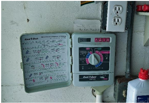
Fig 9.1 East side irrigation system control panel
