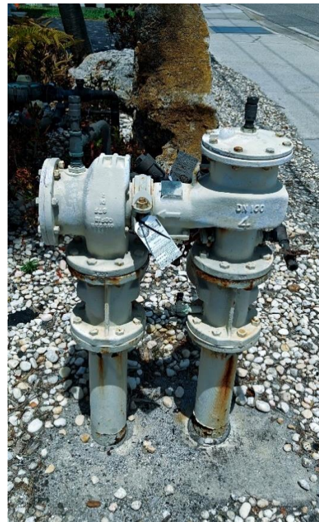
Fig 7.4 Standpipe by street
