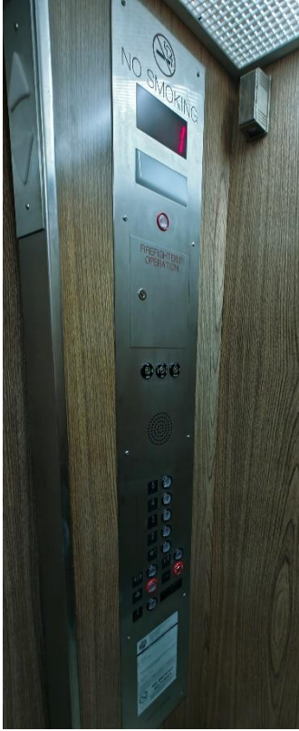
Fig 11.3 Inside elevator panel
