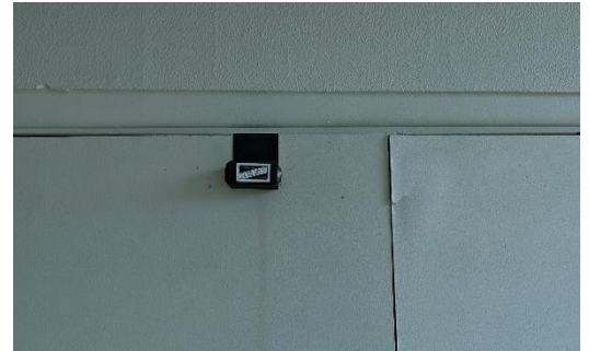
Fig 11.6 Elevator door key box
